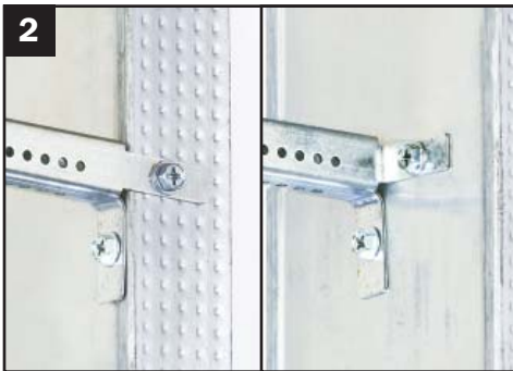
2 Fasten both tabs on each end. Tabs will attach flush with, or inside studs/joists.
